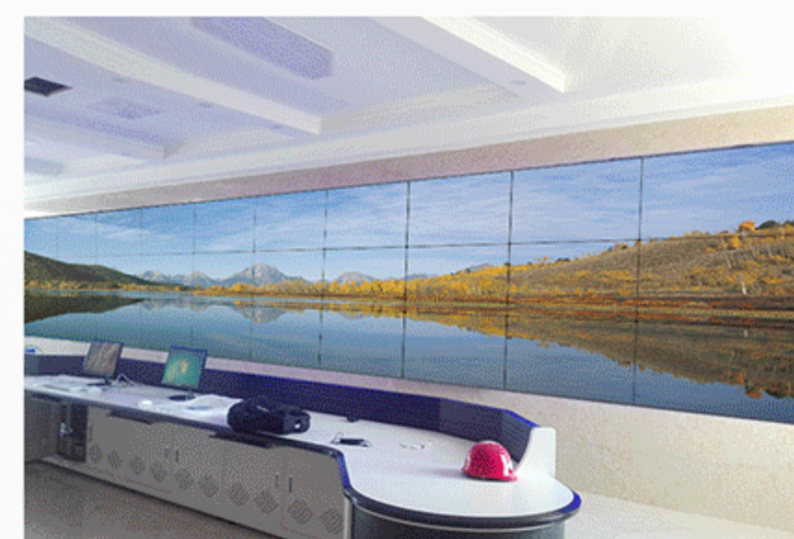
某地区生物天然气厂 Biological gas plant in a region 3x10 55寸拼接 3x10 55 inch video wall
