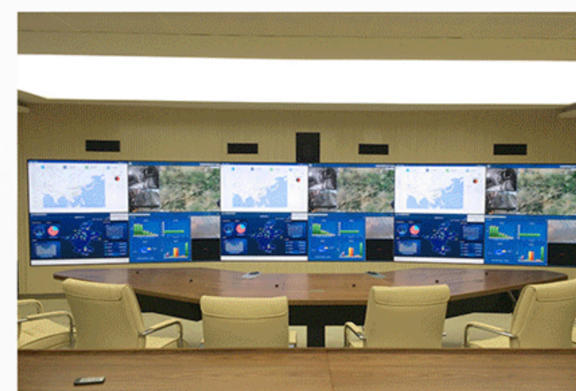
某央企大厦会议室 Conference room of a central enterprise building 2x6 55寸拼接 2x6 55 inch video wall
