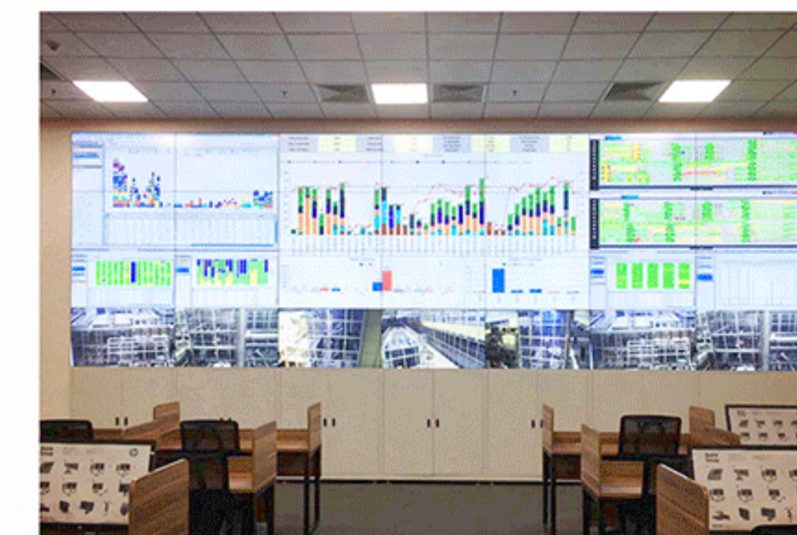
某地工厂 A factory somewhere 4x7 55寸拼接 4x7 55 inch video wall
