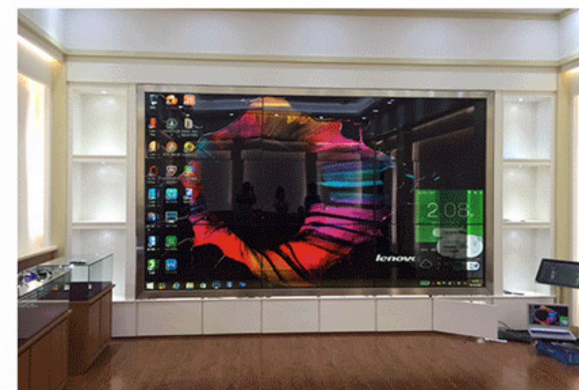
某地区消防支队 Fire brigade in a district 3x3 55寸透明拼接 3x3 55 inch transparent video wall
